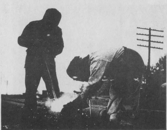
15 To move the oil economically from Leduc field to Nisku railhead an eight-mile pipe line system was constructed. This was extended later to reach Imperial's Edmonton refinery
